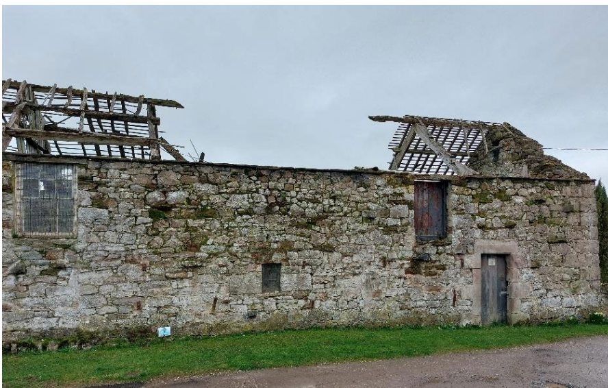
Although derelict, the walls of this barn at Stainton near Penrith are embodied carbon that may be capable of repair, and re-use.
