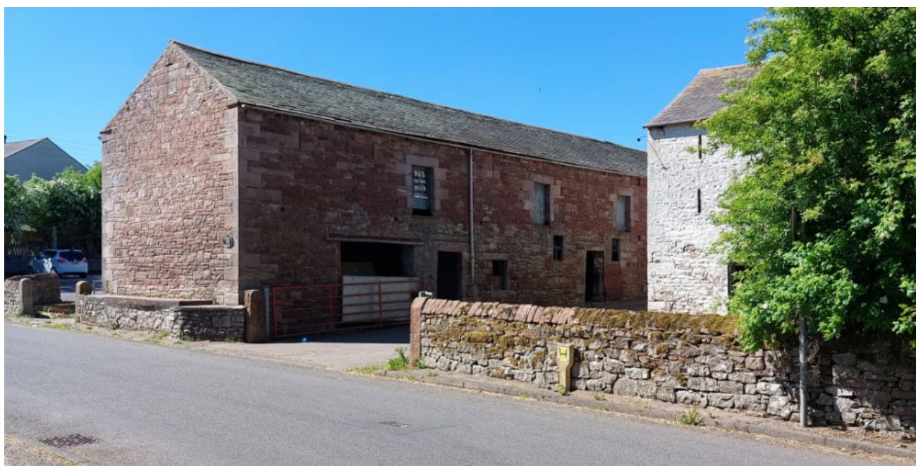
This barn has many different openings on the elevation, but by contrast, the long roof is plain and uninterrupted. A conversion should maintain this aspect of the barn's character and appearance. Skelton.
