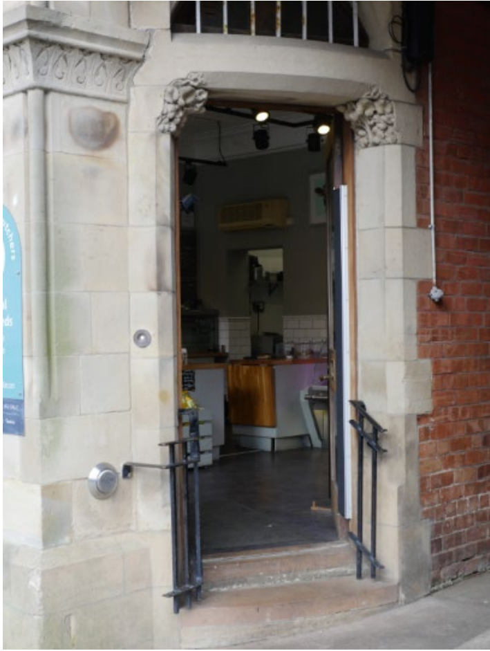
Levelled steps, handrails, a propped open door, and push bell at wheelchair user height are all examples of reasonable adjustments being made to address the floor level change and a heavy door. Appleby.
