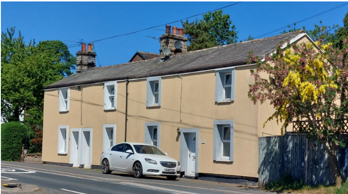
The strongly recessed windows and doors add interest to this elevation and give the walls a sturdy appearance. In this case the additional depth appears to be the result of adding external insulation to the houses. Low Hesket.
