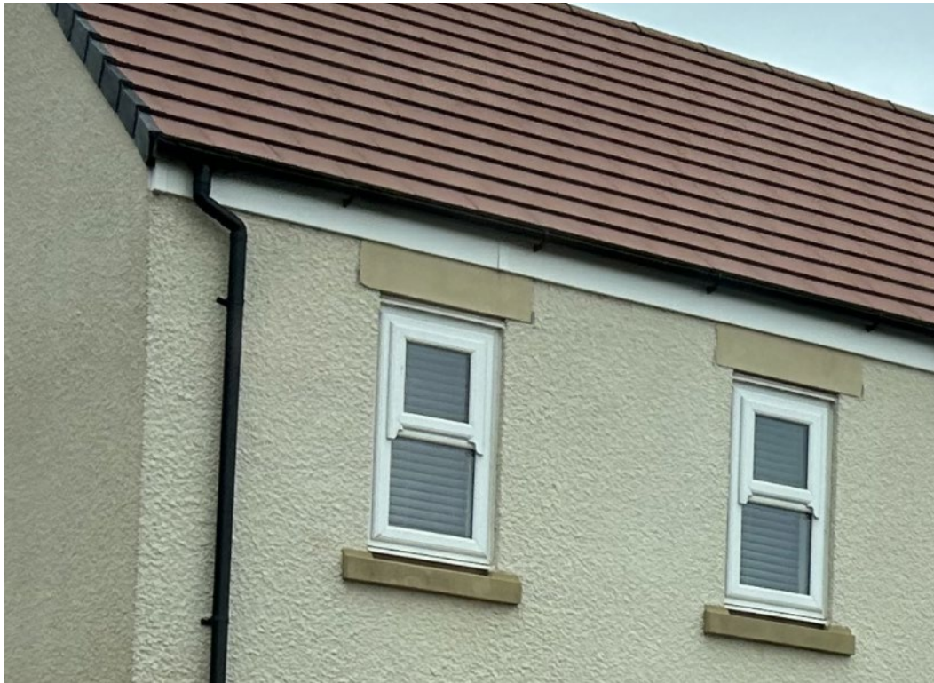
The exterior of this new house is entirely made of materials that are energy intensive (artificial stone sills and lintels and synthetic / cement render) or have short lifespans and will go to landfill (uPVC rainwater goods, fascias and windows). Penrith.
